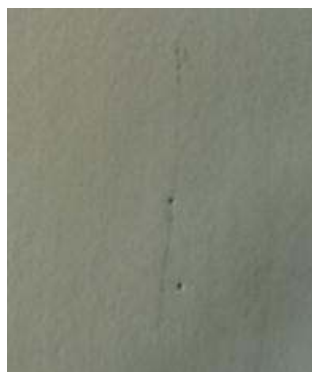
Figure 5: Destructive examination of Defect F in Specimen 4419-02 / BT01
